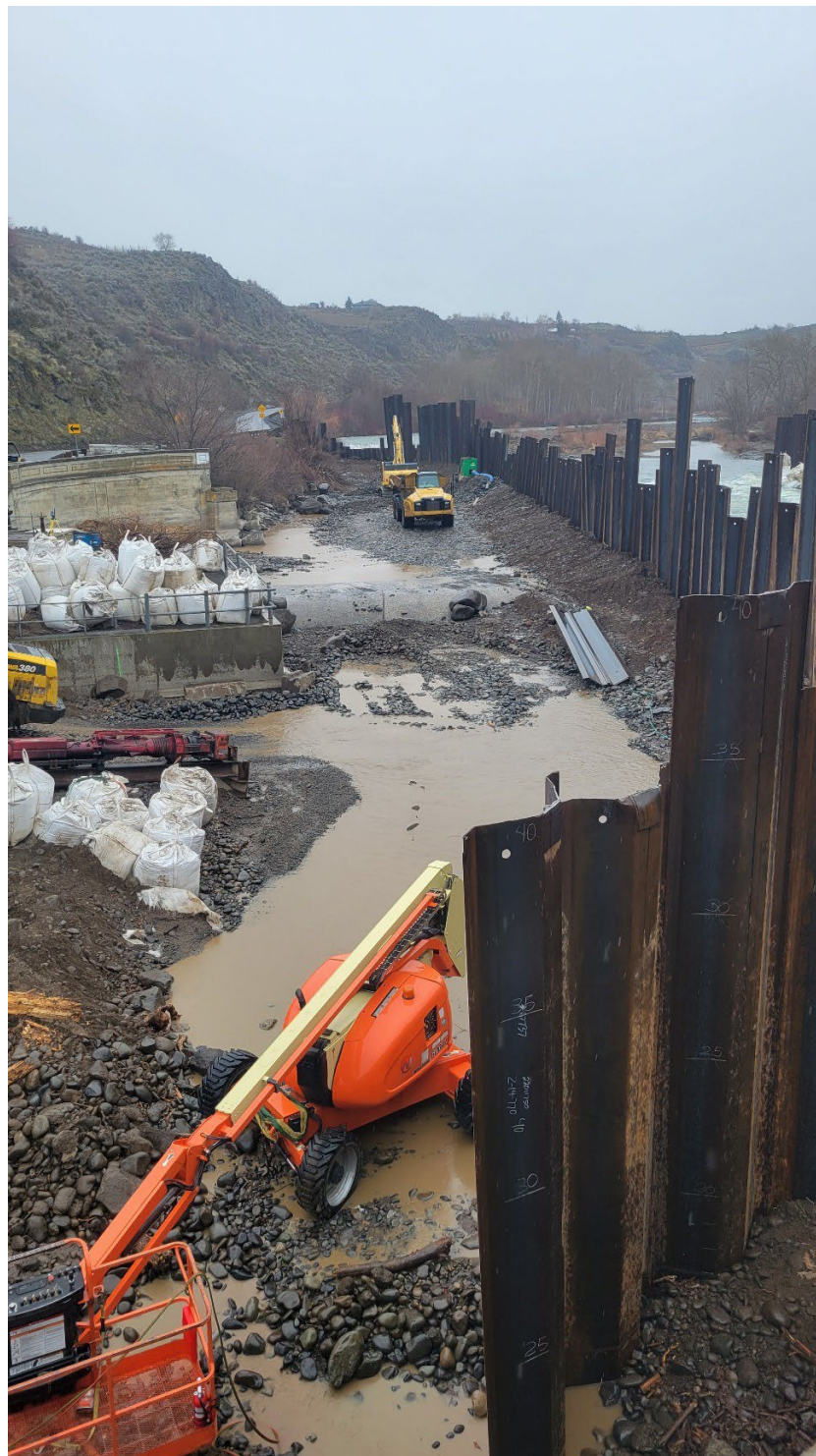
Photo 2. South bank in-water work isolation area for sluiceway and intake work. Area will be isolated behind cofferdams through July 16, 2022.
