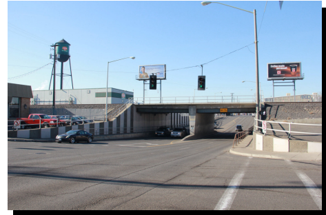
The Walnut Avenue underpass opened in the mid 1950s and was widened in the early 1970s.
