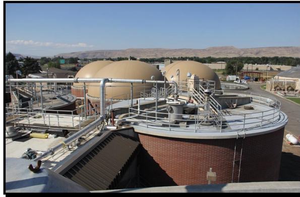
The Yakima Regional Wastewater Treatment Plant has won the 2015 DOE Outstanding Performance Award.
