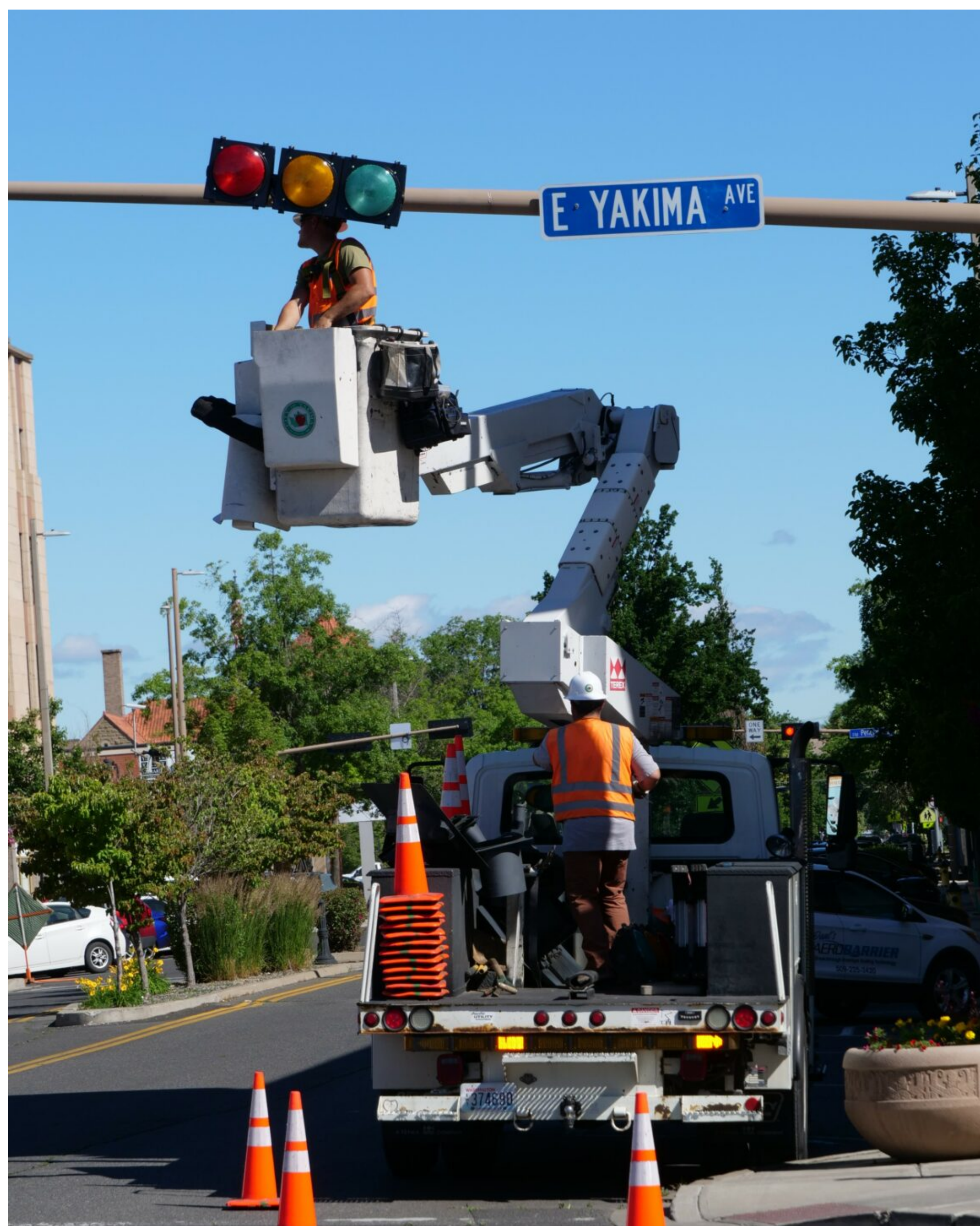
City of Yakima crews are pictured last summer during a series of traffic signal upgrades along Yakima Avenue. Crews are upgrading additional signals this summer.
