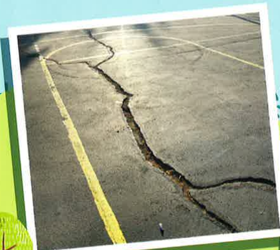
Hazardous cracks and uneven surfaces
