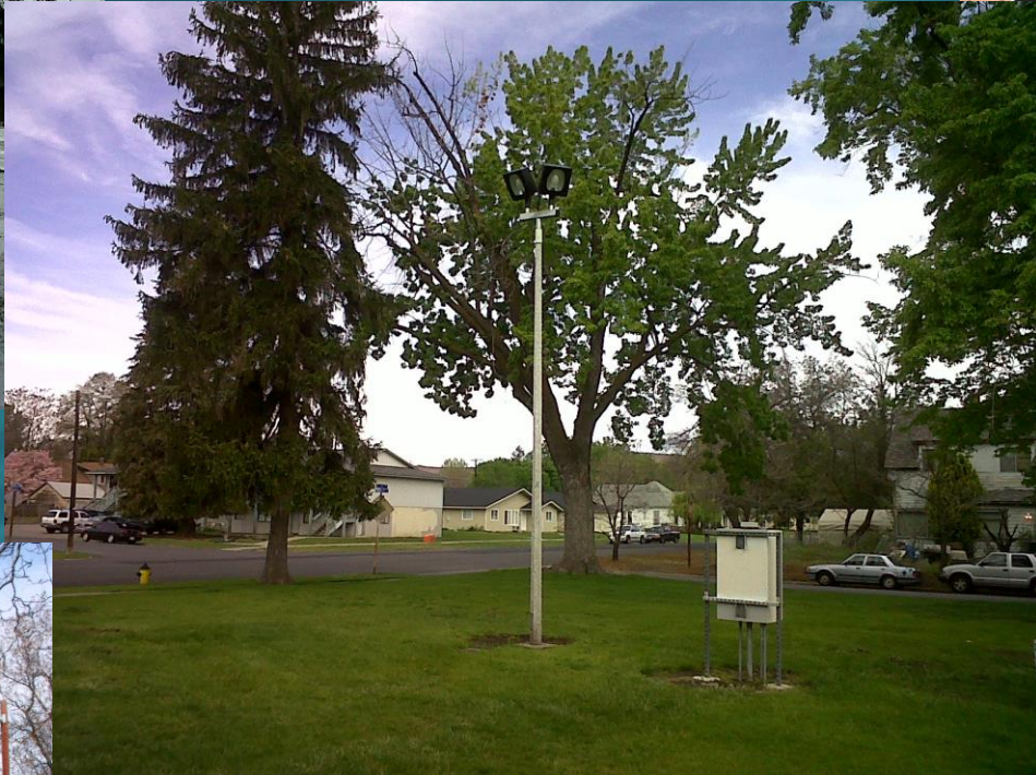
Security Lighting Installed - 2018
