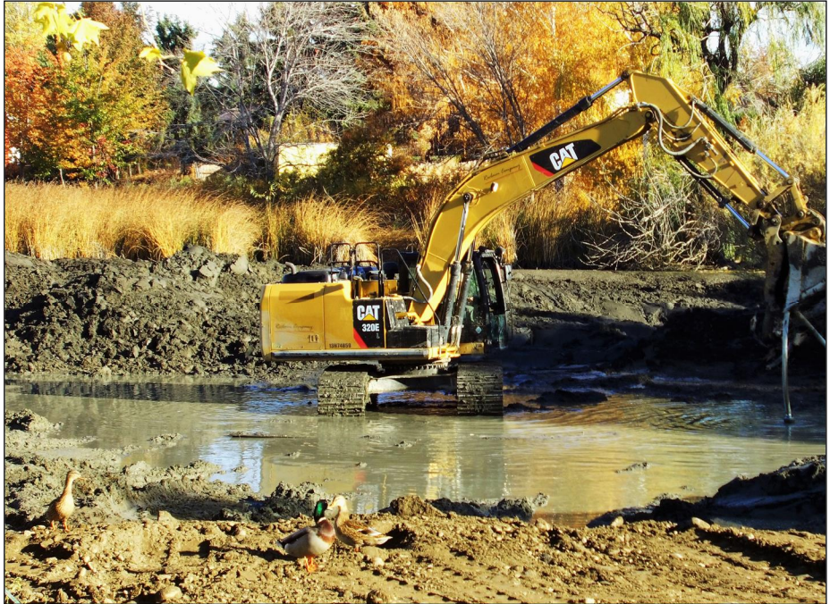
Improvements now underway at the Randall Park pond will ensure the pond's longevity for duck and human visitors for years to come.
