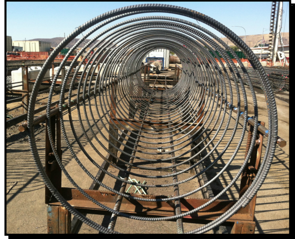
Circular steel cages made from rebar are being used to form reinforced concrete columns for underpass retaining walls.
