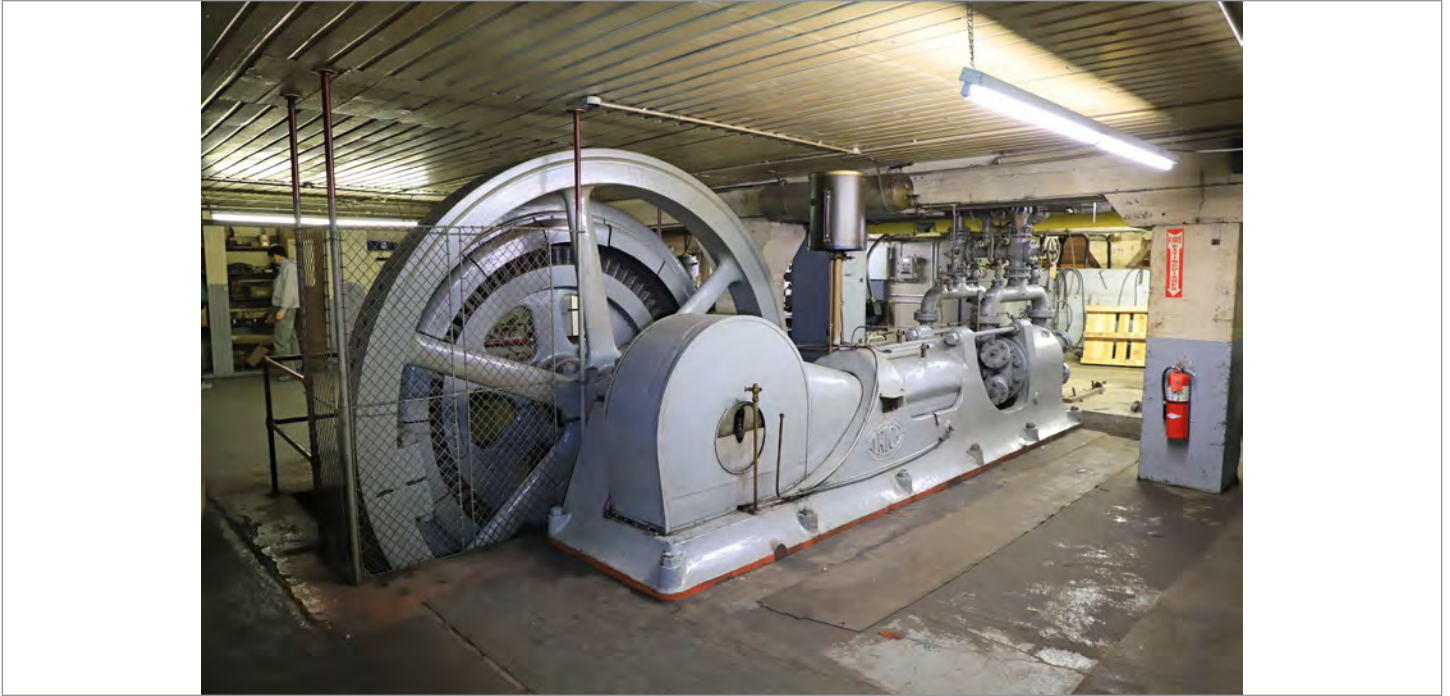
WA_Yakima County_Fruit Row_0025. Ammonia compressor in basement of 201 N First Avenue.
